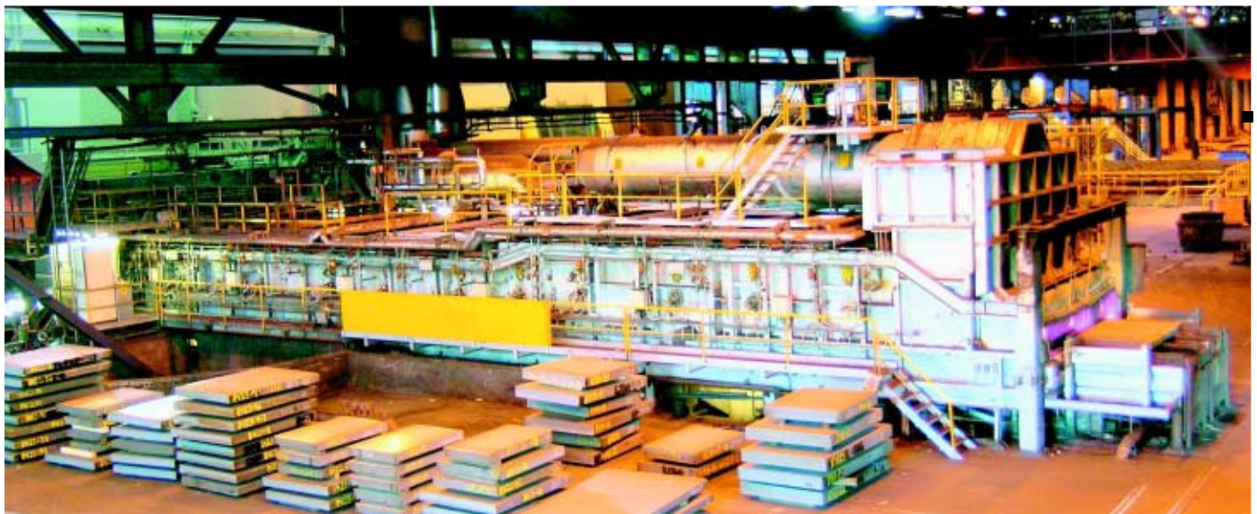
The turnkey flameless oxyfuel project in the walking beam furnace at Outokumpu Stainless, Degerfors site, resulted in 40-50% more heating capacity and 25% reduced specific fuel consumption compared to the earlier airfuel burners and recuperator.
